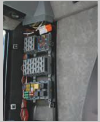
The electric fuses panel.
